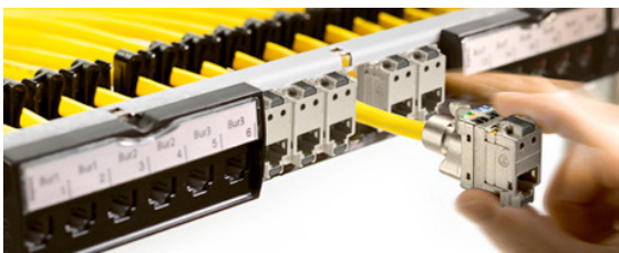
Εικ.14 Patch panel UTP (Courtesy Legrand)
